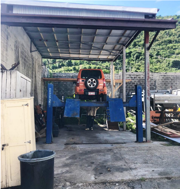
The Mechanic Shop received a face lift and the reconstruction of the roofs over both the Two Post and Four Post lifts.
