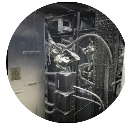
Figure 2 & 3: Fire at the Henry Wilfred Smith Power Station
